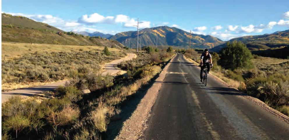
Two miles of dual-surface trail was constructed in 2014 above Woody Creek. The construction of fully separated hard and soft surfaces is the goal where possible. Cindy Klob photo
