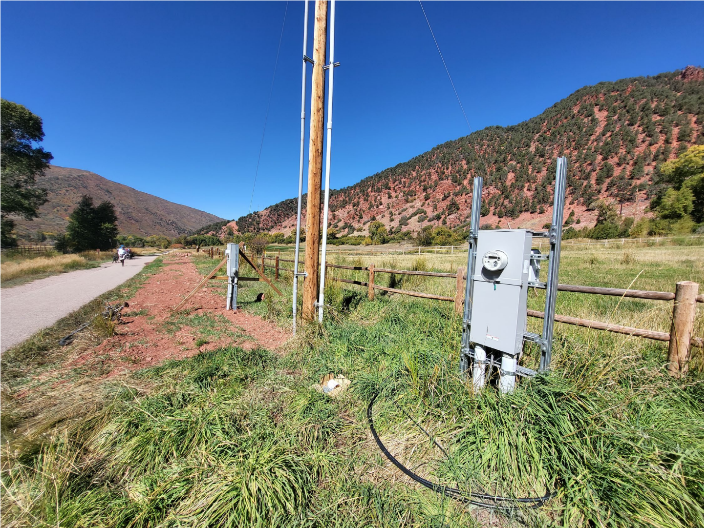
Photo – electrical system
