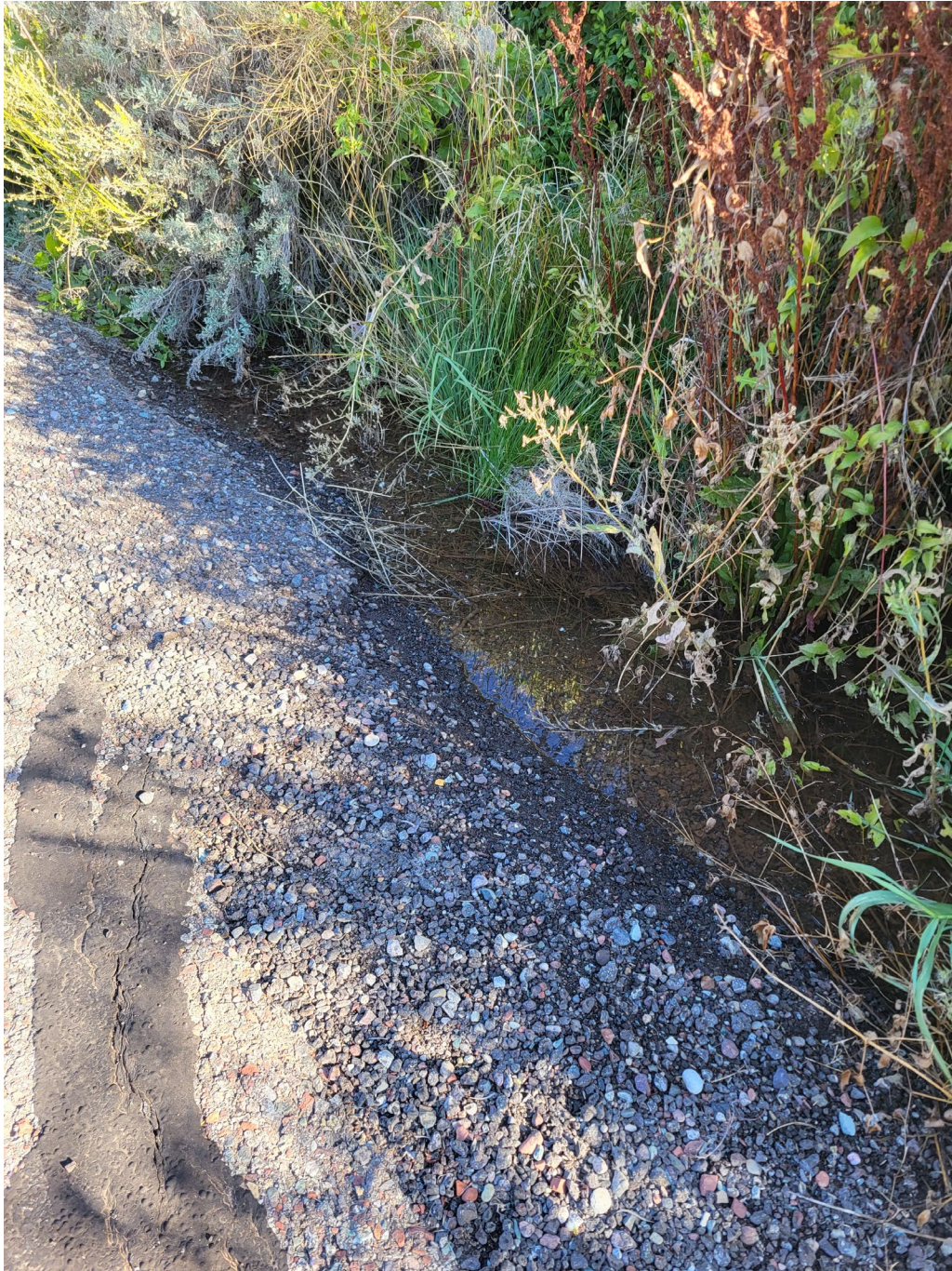
Photo – location #2 water along RGT shoulder from Thompson Glen Ditch
