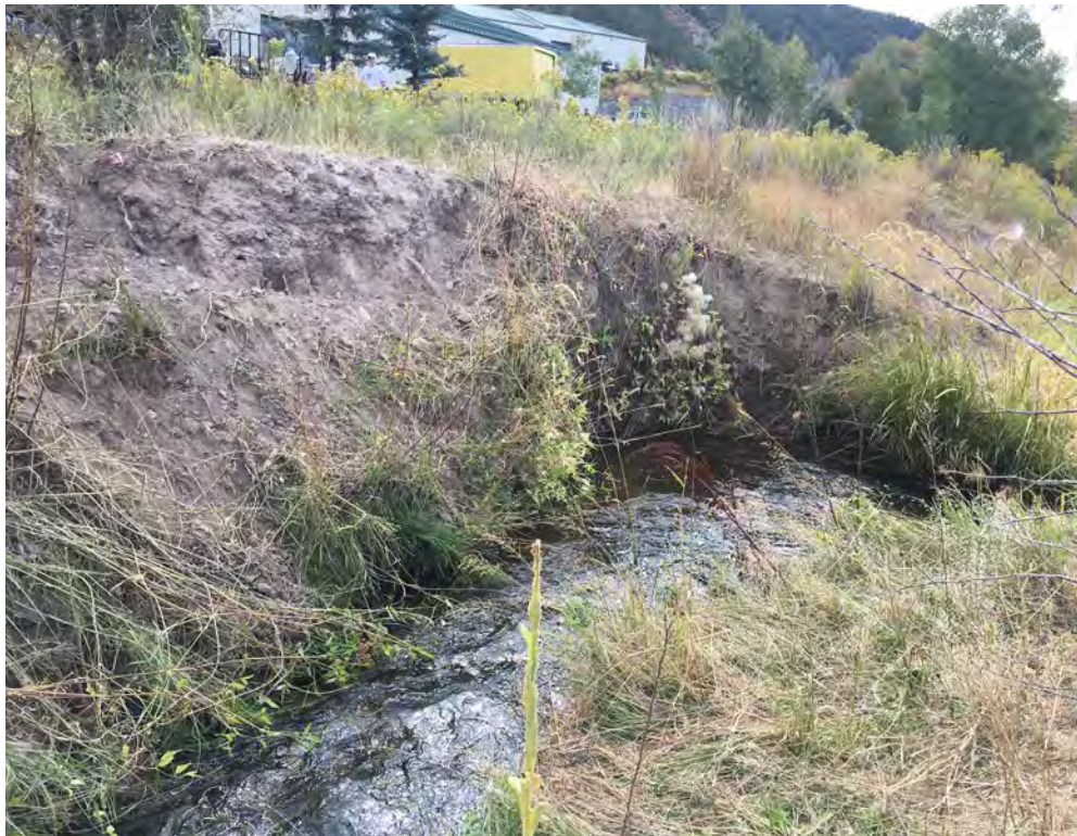
4. View looking N at area of significant impairment. Evidence of erosion and poor vegetation establishment along steep bank of irrigation ditch.
