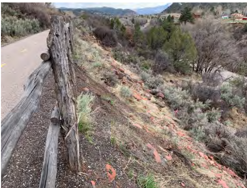
Figure 2 - Significant impairment conditions (MM 365.75)
