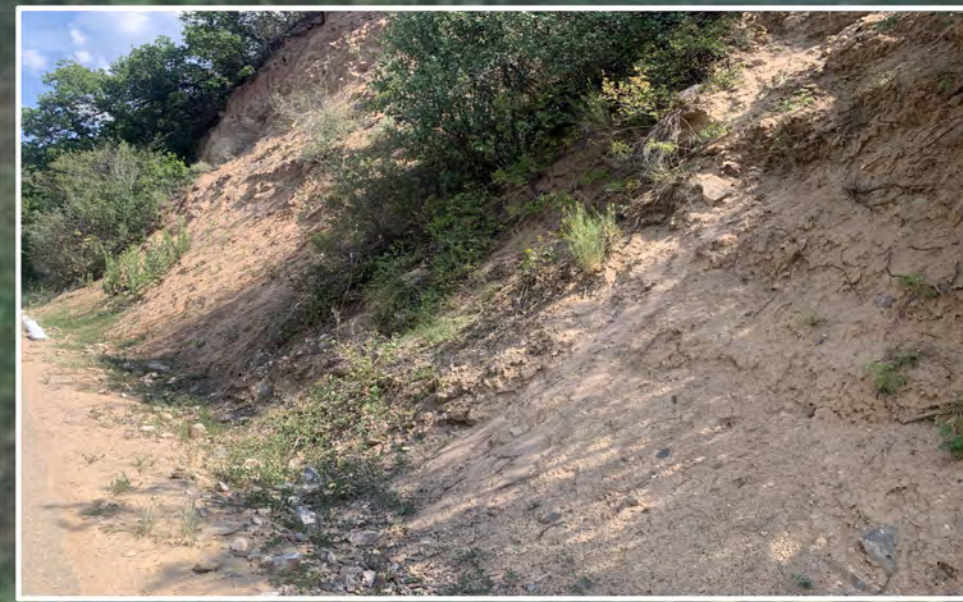
View Looking east (up valley) at restoration priority area 1, MM 376.2. Steep slopes and poor vegetation establishment with potential for sever erosion activity. Recommend using the aggressive erosion control seed mix #4 with Hydraulic erosion control to stabilize slopes
