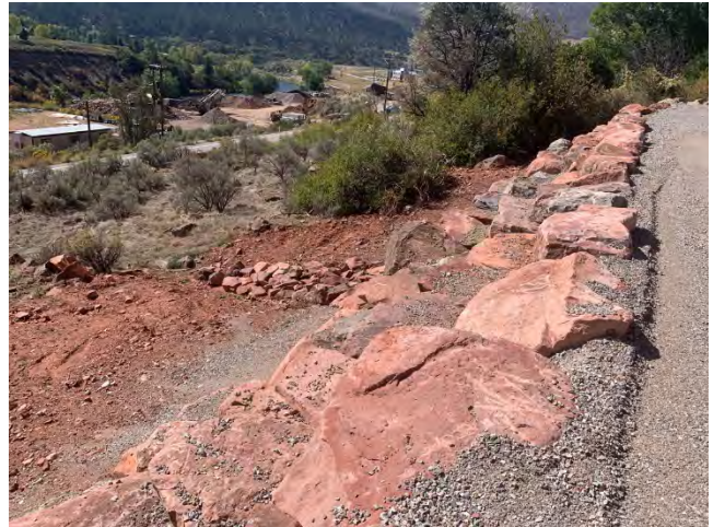
Figure 9 View looking NW at Priority 1. Bare soils from construction disturbances
