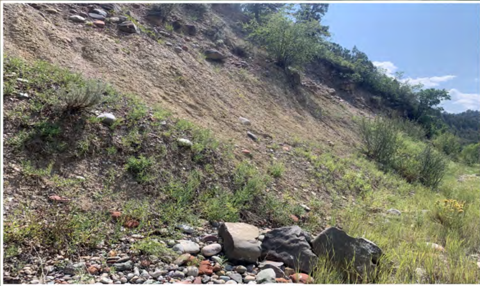
View Looking west (down valley) at restoration priority area 2, MM 376.9. Steep slopes and poor vegetation establishment with potential for severe erosion activity. Recommend using the aggressive erosion control seed mix #4 with Hydraulic erosion control to stabilize slopes
