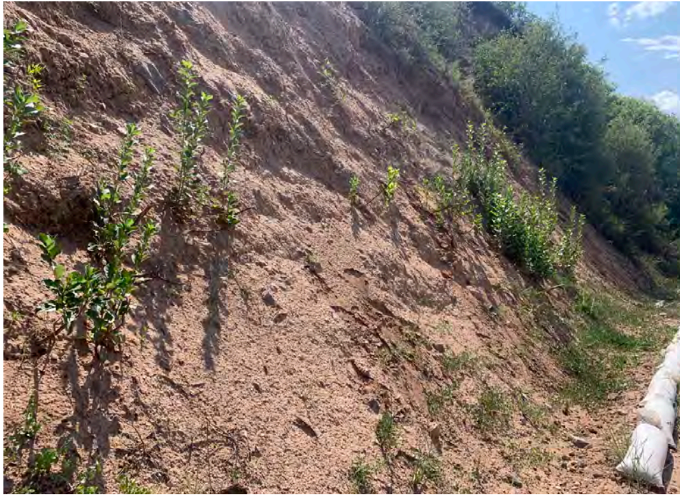
1. View looking west at significant impairment area. Steep bank with poor vegetation establishment with high erosion potential and issues.
