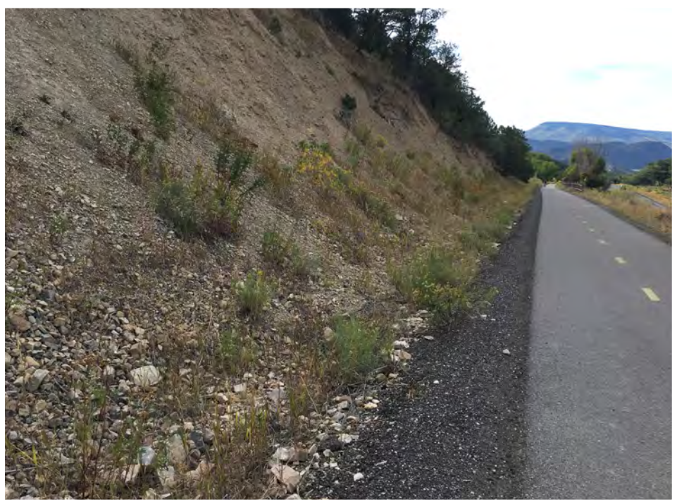
View looking west along restoration priority area 1, MP 374. Steep slopes and lack of vegetation with evidence of severe erosion activity. Recommended restoration activities include using the aggressive erosion control seed mix 4 on the slopes with a Hydraulic erosion control product to stabilize slopes. The toe of the slope should be seeded using the #2 seed mix for sagebrush shrublands.
