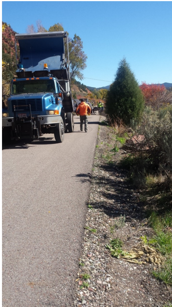
Photo – Before shoulder repairs were complete, lip off the edge of asphalt is very evident.
