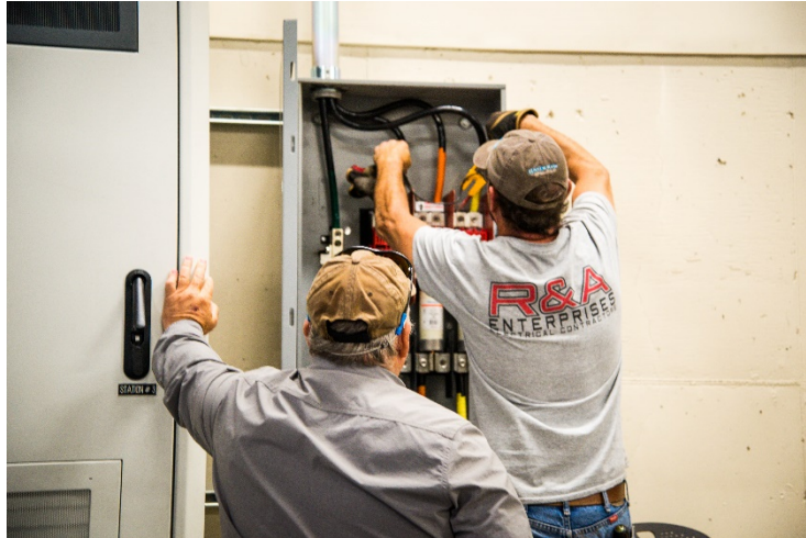
Contractors put the finishing touches on BEB charging equipment
