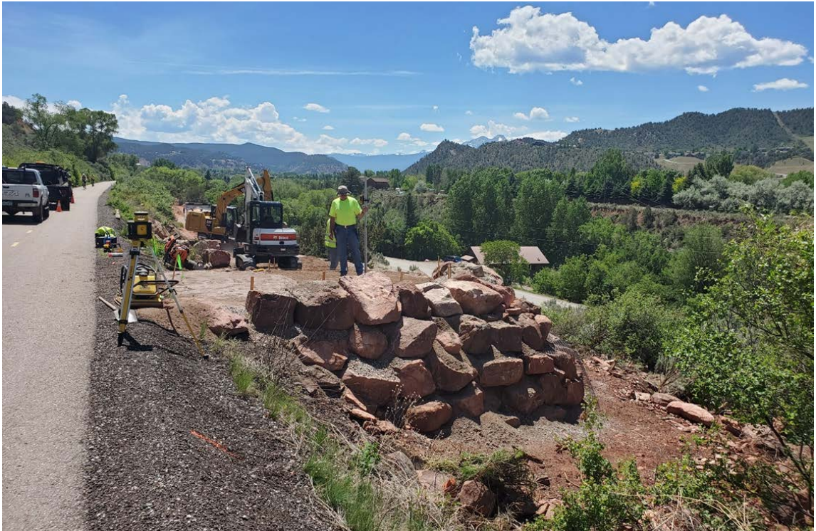
Photo 1 – Safe Routes to School: Riverview Trail. Construction activities at the “tie-in” to the Rio Grande Trail
