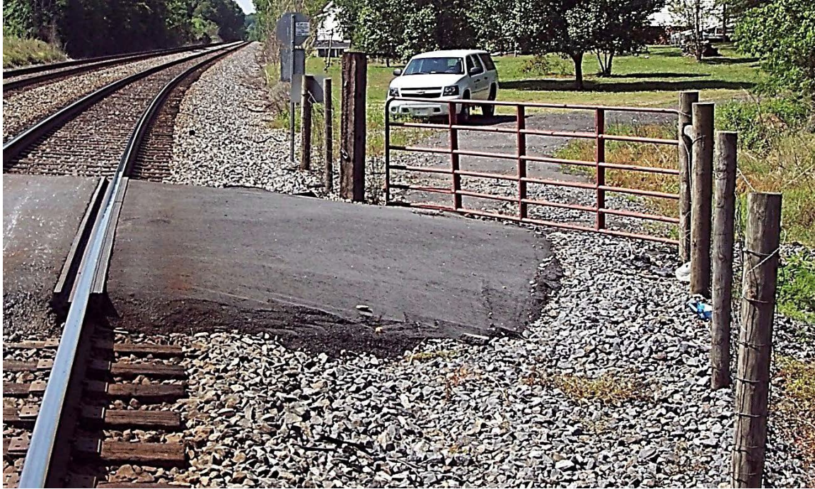
Exhibit 18 – Tubular Steel Right-of-way Barrier Gate
